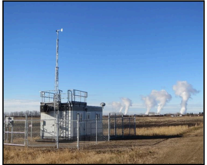
Figure SEQ Figure \* ARABIC 12: Scotford South Station
