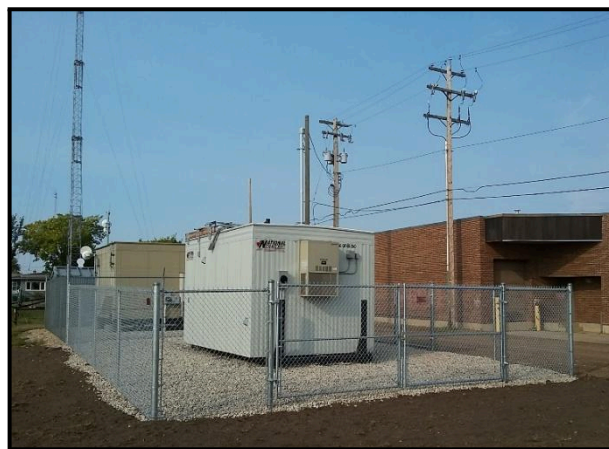
Figure SEQ Figure \* ARABIC 10: Redwater Station
